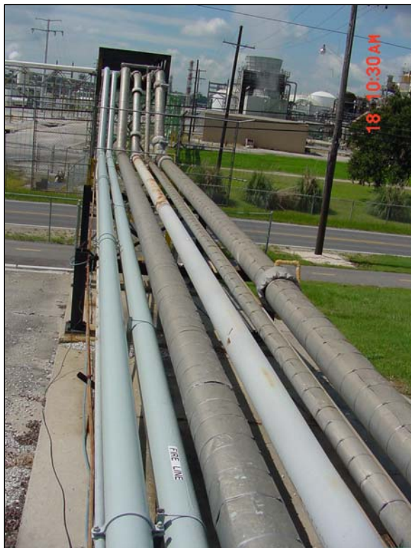
Figure 4.1.1 Unlabeled pipelines over Mississippi River levee
